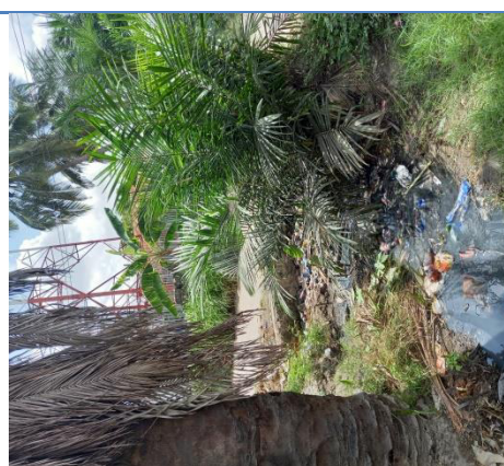
Figure 3.4 B: Street Terrace Blocked due to Debris Contaminated with Plastics.
